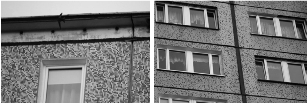
Figure 1. Main places in panel buildings where swifts build nests: ventilation holes in attics (left) and crevices between panels (right)
