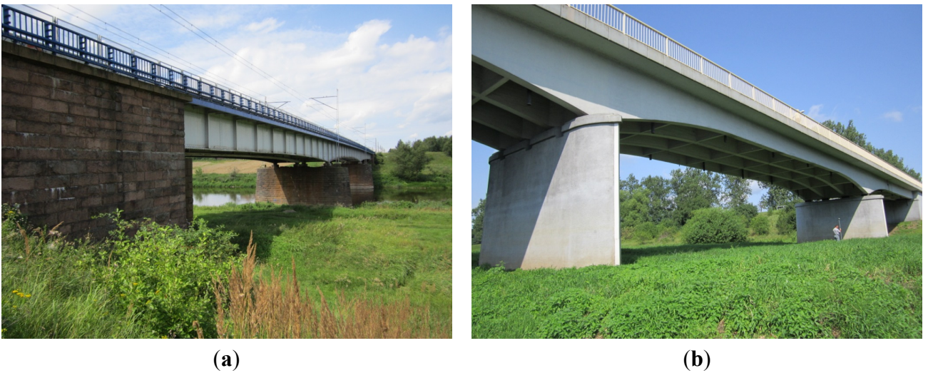
Figure 2. The existing bridges located in the town of Wronki: (a) railroad bridge in km 168 + 773 (downstream); (b) road bridge in km 169 + 871 (upstream) [8].
